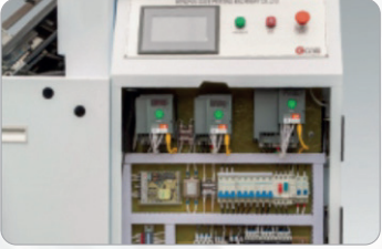
PLC触摸屏，施耐德电器 PLC touch screen, Schneider electrical
